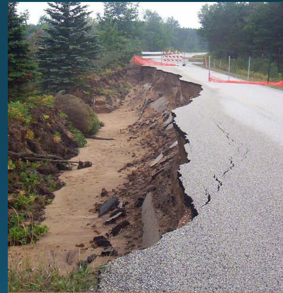
Road damage on Lake Michigan Drive near Ludington due to runoff from the June 12, 2008 storm that dumped 10 inches of rain in 12 hours. Photo: Chris Pierce
