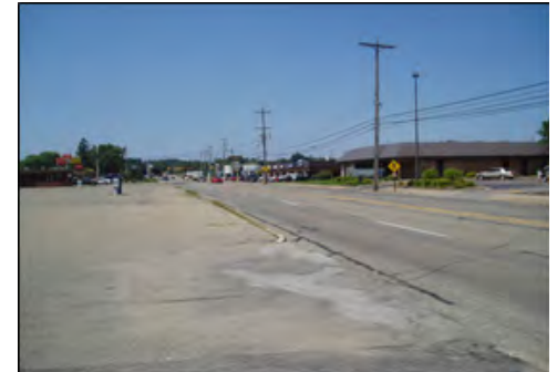
Successive layers of pavement have nearly overtopped the curb, further exacerbating access control in this area.
